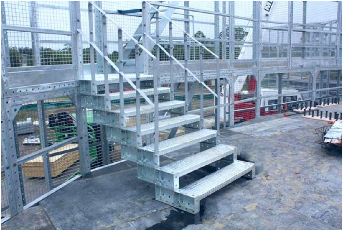
Figure 1 - Example of super scaffolding to act as edge protection this would be set up on top of rock surface.
